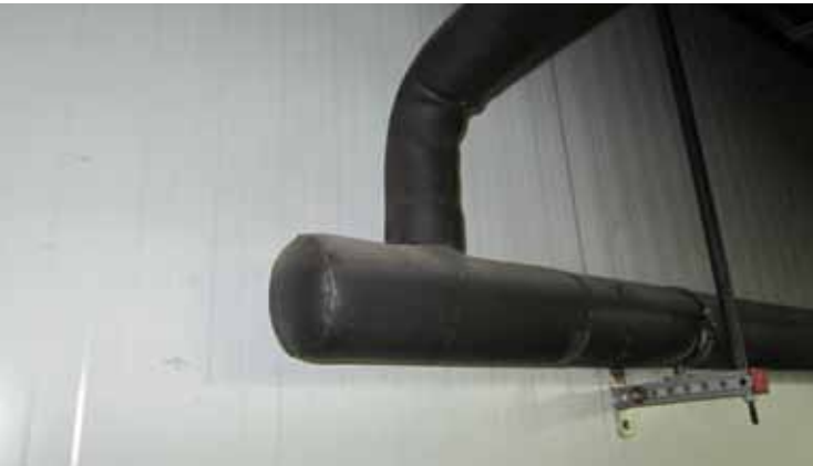
Figure 16. Pipe insulation in good conditions.
