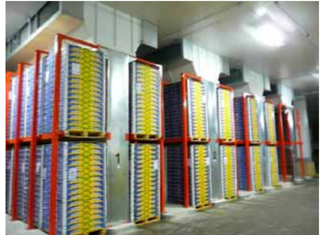
Figure 4. Vertical air-flow pre-coolers reduce pre-cooling time, which increases fruit and vegetables shelf life and quality, and save energy costs.
